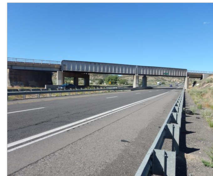
Existing bridge 6226 carries the BNSF railroad tracks over I-40 at MP 94.77. Condition ratings and other data for this bridge were not available, and horizontal clearances are limited by the piers.
