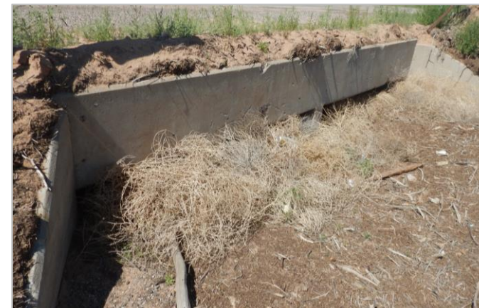
CBC clogged with sediment at MP 31.7.
