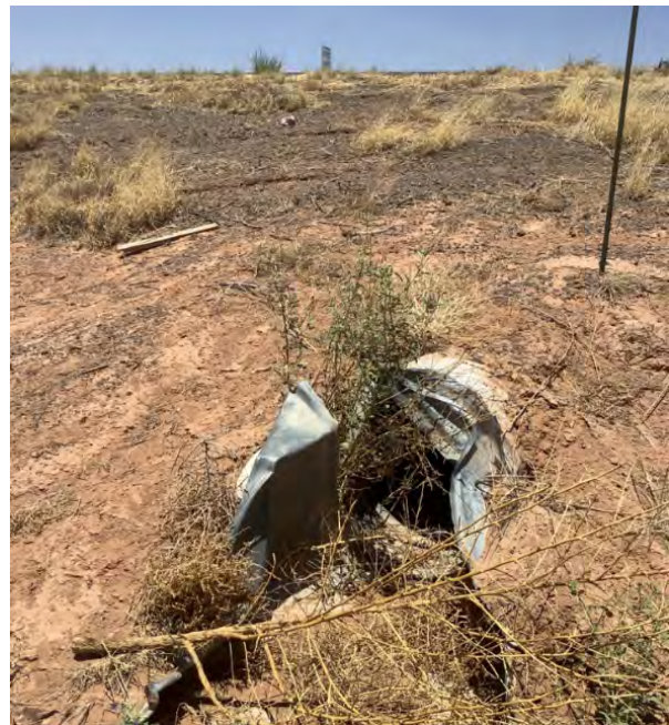
Example of a Heavily Damage Metal Pipe
