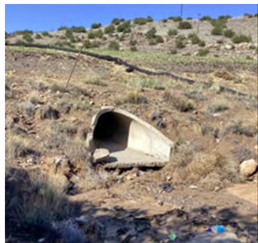
Example of a Broken Concrete End Section
