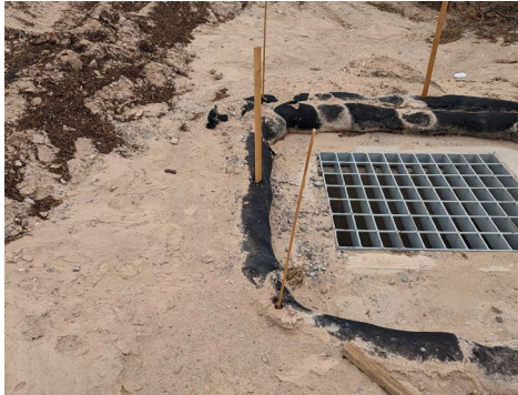
Correct: Mulch socks located to protect inlet, overlapping mulch socks Incorrect: Sediment collected behind mulch sock, stakes damaged, 2" x 2" stakes should be used
