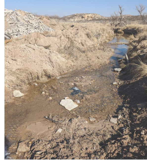
Correct: Mulch socks staked at base of debris pile Incorrect: Unstabilized slope, construction debris in waterway, debris pile within buffer zone of waterway
