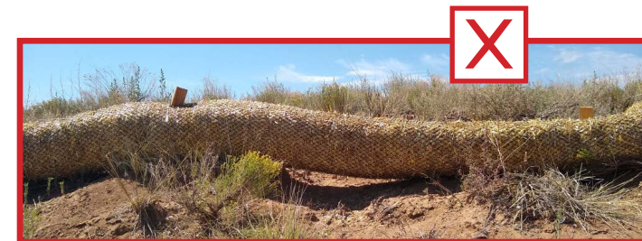
There should never be a gap between the ground and the bottom of a mulch sock
