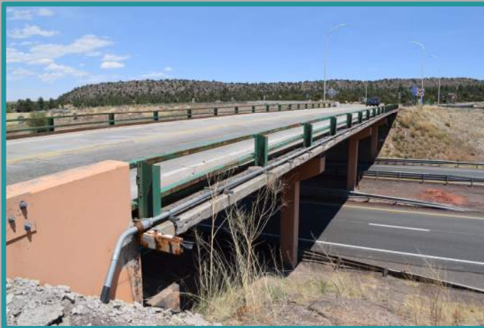
View of South Bridge Elevation with Substandard Bridge Railing
