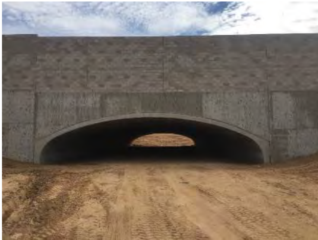
Figure D-25. Arch wildlife underpass on Arizona's six-lane SR 77. Wildlife have used it over 5,000 times to pass beneath the highway (photo credit: J. Gagnon).
