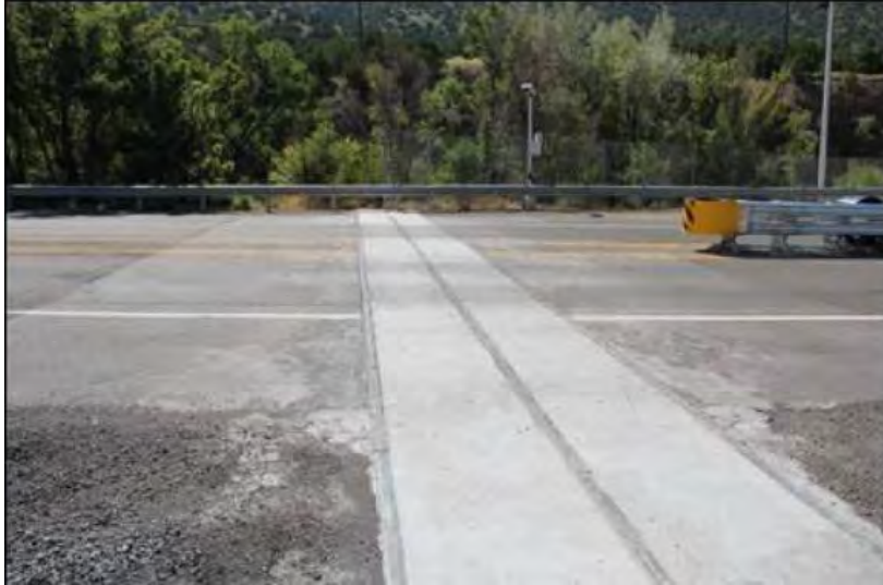
Figure A-8. Tijeras Canyon Safe Passage Project electrified concrete barriers at NM 333 wildlife crosswalk (photo credit: AZGFD).
