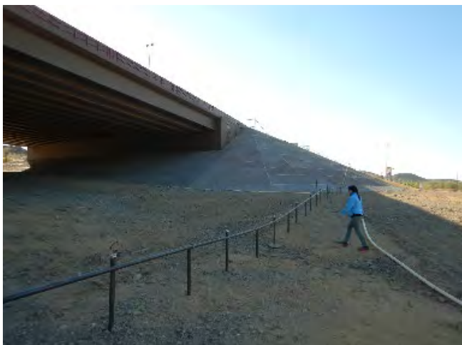
Figure D-35. Arizona placed a steel rail fence at a wildlife underpass structure to deter motorized vehicle use (photo credit: AZGFD).
