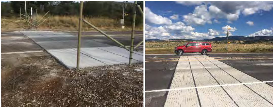
Figure D-47. Electrified barriers installed along SR 260 in Arizona (left) and along US 550 in New Mexico (right) to keep elk and deer out of the right-of-way (photo credit: AZGFD).
