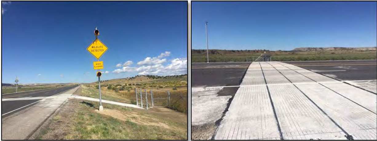
Figure A-27. Driver warning signs and electric pavement at fence end on US 550 (photo credit: AZGFD).
