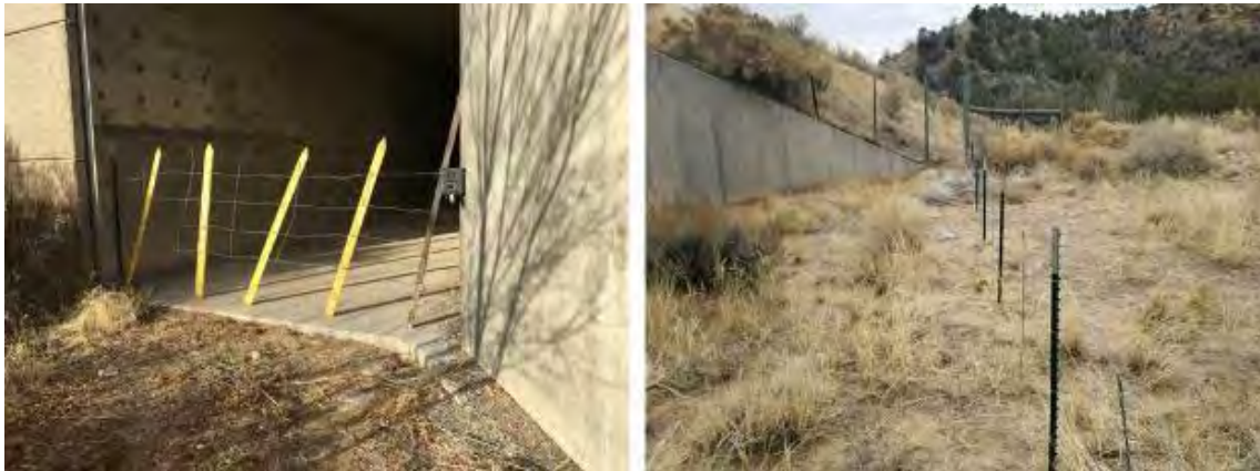
Figure D-9. Fence placed at entrance of concrete box culvert under US 550 near Aztec, New Mexico (left) (only four mule deer successfully crossed), and NMDOT adapted fence placed away from concrete box culvert entrance to enhance mule deer movement while containing cattle (right) (741 successful mule deer crossings) (photo credits: J. Gagnon, AZGFD).
