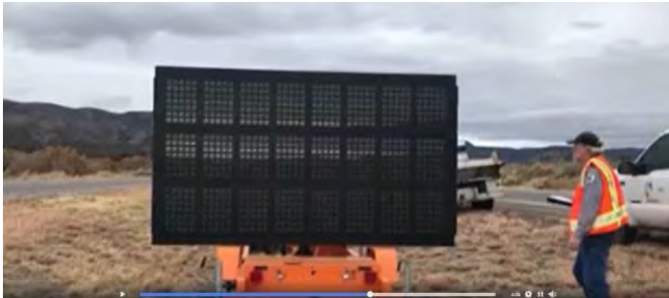
Figure D-51. M. Watson of NMDGF installs driver warning variable message board with NMDOT maintenance personnel (photo credit: NMDGF).
