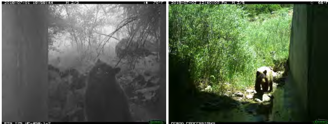
Figure D-30. In New Mexico, black bear have regularly used existing box culverts to cross under I-25 near Raton (photo credit: AZGFD, NMDOT).
