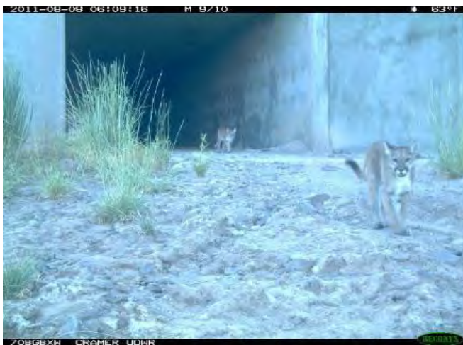
Figure D-29. Cougars use ranch operations concrete box culvert under I-70 in Utah (photo credit: P. Cramer, UDOT, and UDWR).
