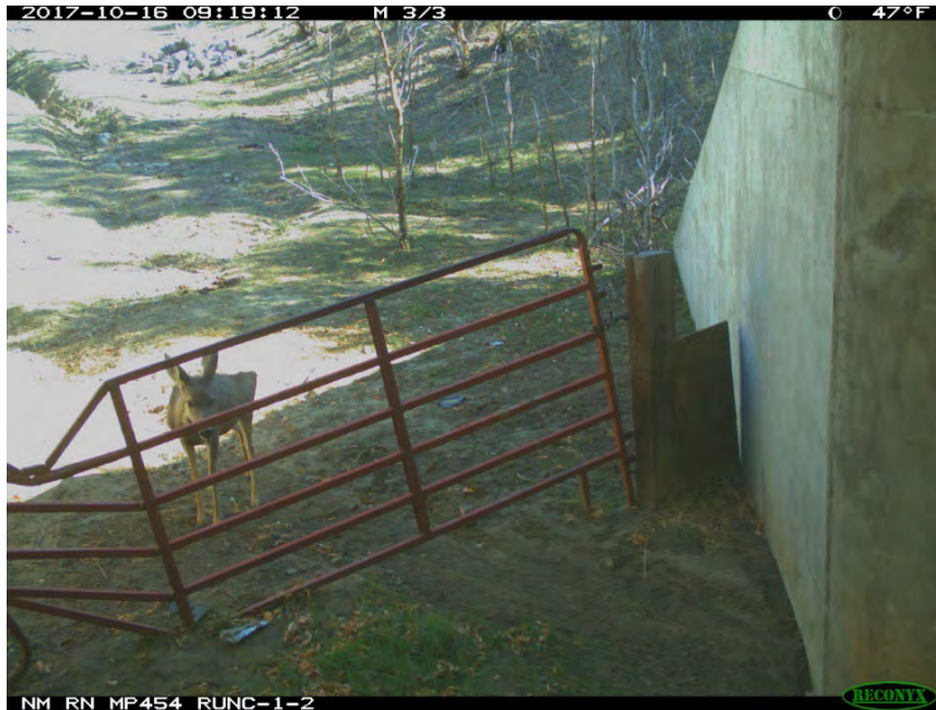
Figure A-16. Gate placed by landowner on box culvert to keep livestock from using culvert (photo credit: AZGFD, NMDOT).
