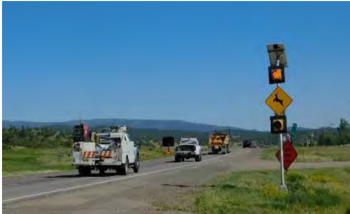
Figure D-49. Warning sign with flashing yellow lights in Chama, New Mexico (photo credit: P. Cramer).
