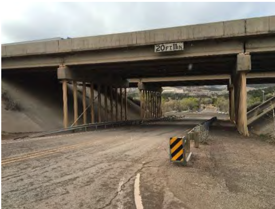
Figure D-4. Tijeras Canyon retrofit of public school interchange under I-40; no known wildlife use (photo credit: J. Gagnon, AZGFD).
